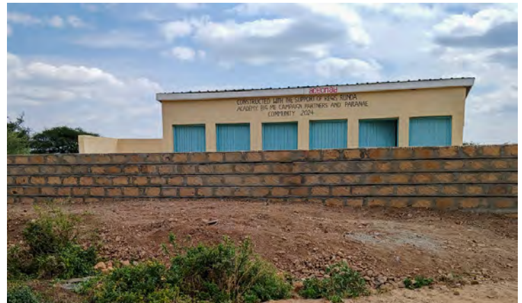
The six-door toilet block constructed with support from Regis Runda Academy, through the BigMe Campaign.
